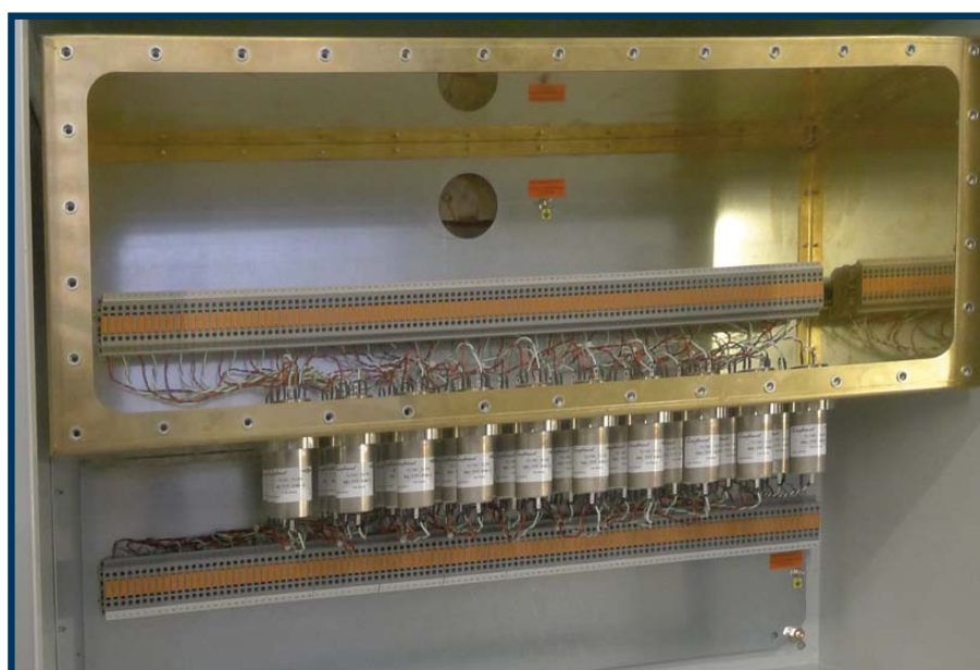
Inside of AAA cabinet
